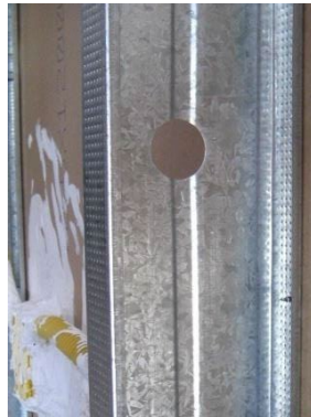
Figure 13: Opening in frame for passage of plumbing or conduits Source: personal archive of Verniz (2010).
