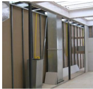
Figure 11: Thicker internal walls for passing air-conditioning components Source: personal archive of Verniz (2010).
