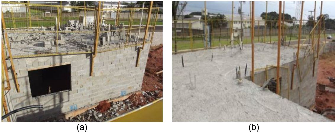
Figure 1: Construction safety railing embedded in structural masonry, and poor fixation of safety elements
