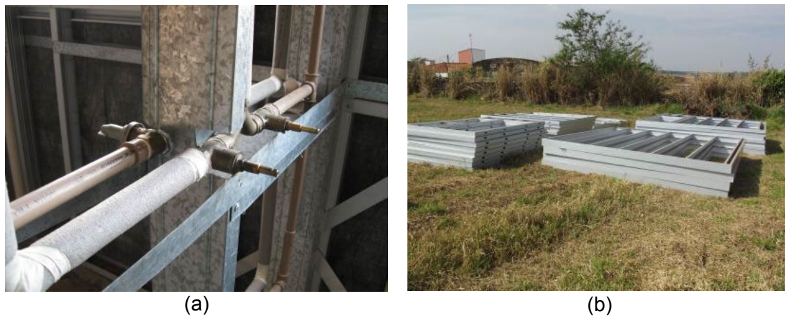
Figure 4: Cuts in structural struts of the light steel frame and inappropriate storage of structural elements of the same system
