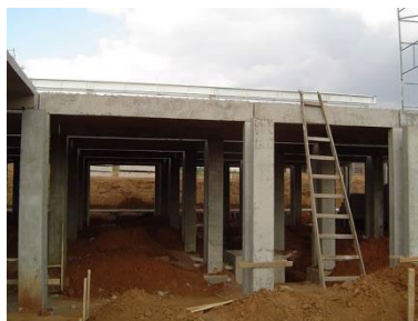
Figure 7: Cast in place concrete columns and slabs Source: personal archive of Fabricio (2005).
