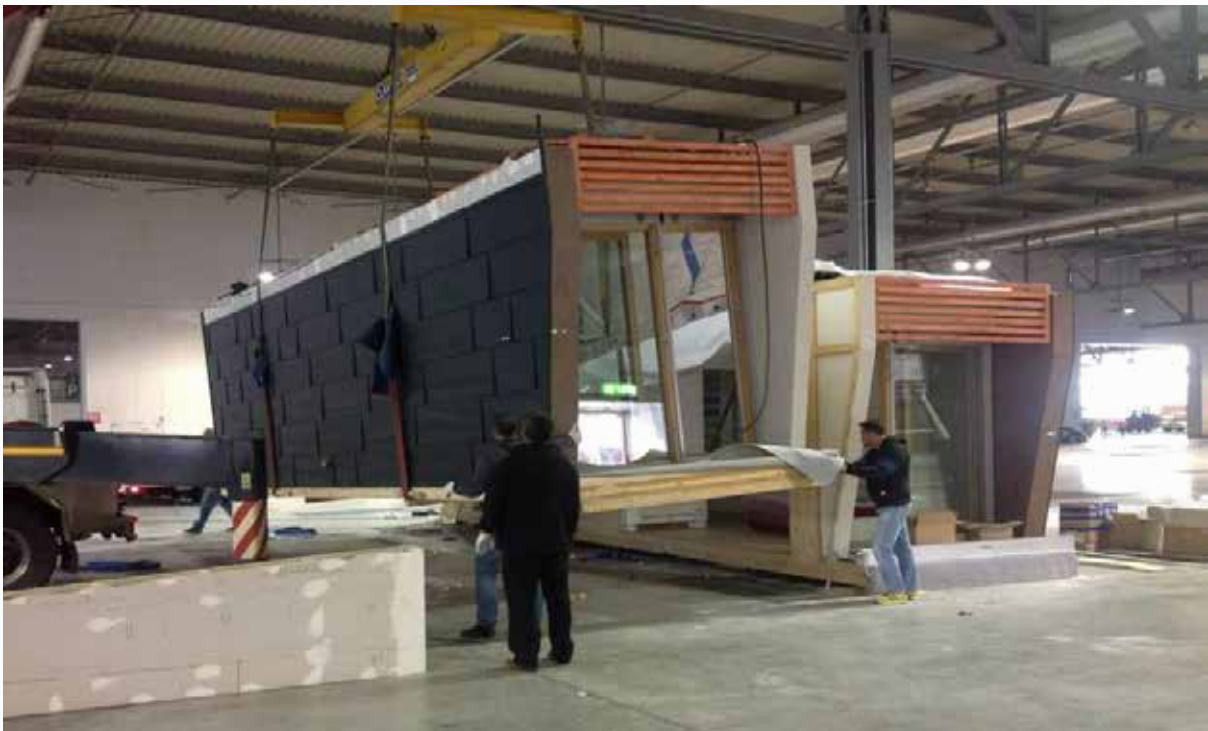
Figure1: The prototype of the modular habitative unit built with two basic modular modules
