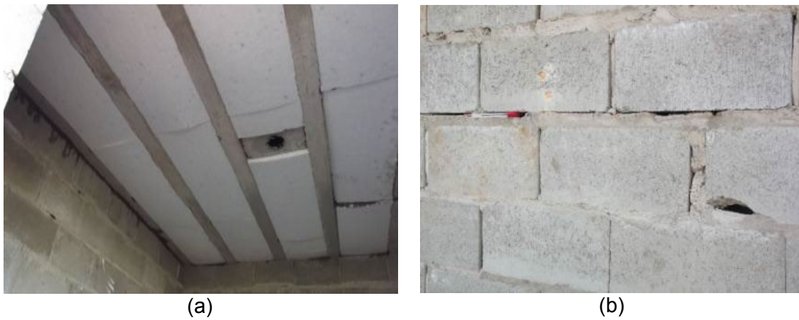
Figure 2: Poor quality slab and joint EPS filler without thickness control in structural masonry walls
