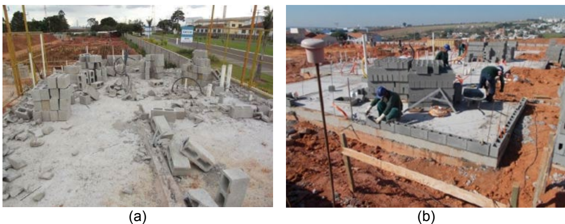
Figure 3: Excessive waste of structural blocks in the slab, and traditional labor-intensive construction site
