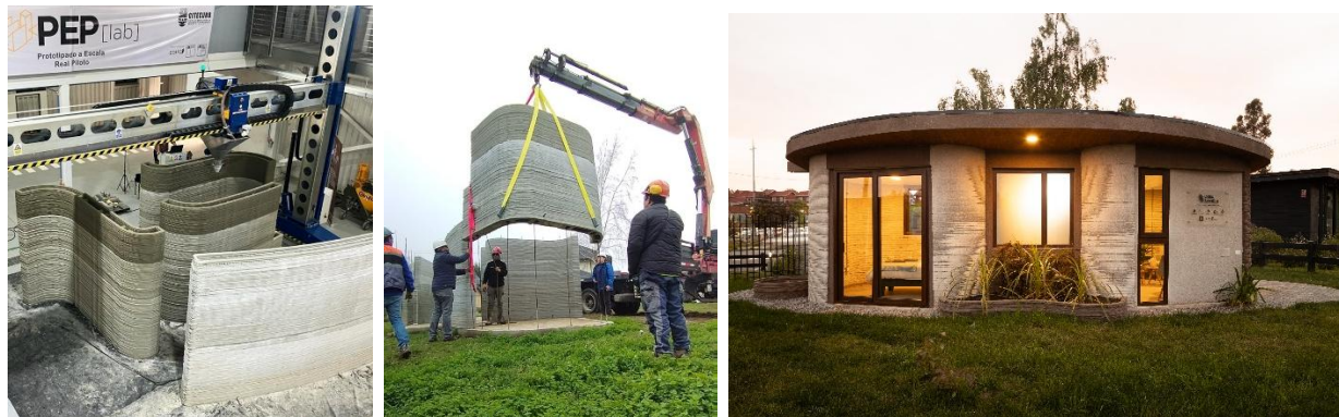
Figure 1: Prototype Construction; Left: Printing of walls in university lab; Center: Assembly of walls on-site; Right: Prototype executed
